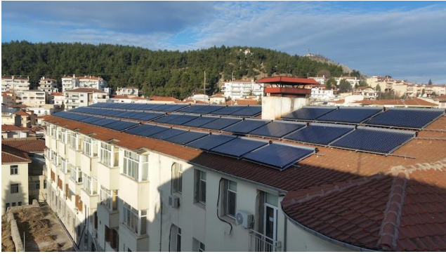
Image 2: Solar collectors in Mamatseio Hospital
