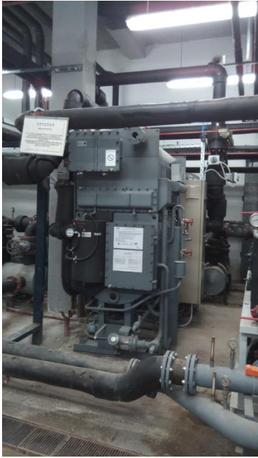
Image 8: Absorption chiller at Mpodosakeio Hospital
