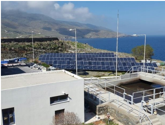
Image 4: PV at the sewage plant of the Municipality of Andros
