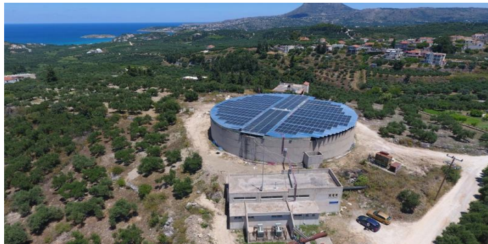
Image 10: Installed PVs on the tank top and the nearby pump house
