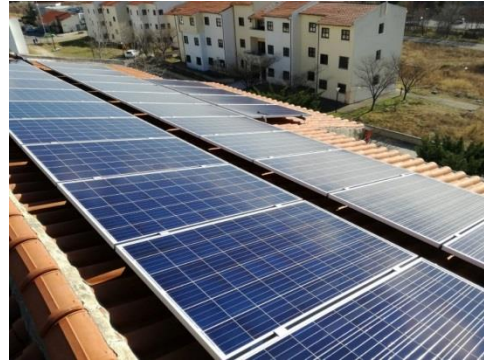
Image 3: PV power station in Democritus University of Thrace
