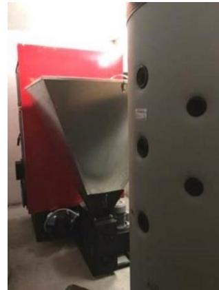
Image 5: Biomass Boiler and feeding system in Alexandroupolis
